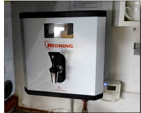
Kitchen water heater
